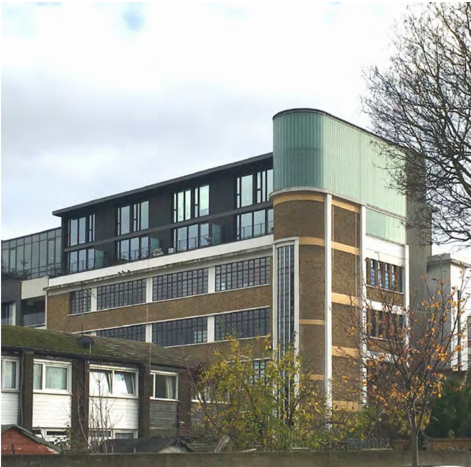
Figure 4.22a: An example of additional storeys being added to an existing building historic example of additional storeys being added toto provide new homes.
