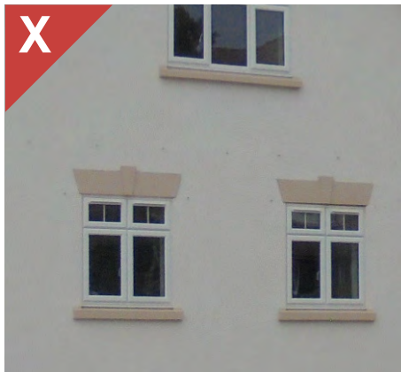
Figure 2.25b: Shallow reveals can result in a poor appearance that lacks depth and windows appear as if they are stuck on. Shallow reveals should generally only be used where they are part of a compelling design.
