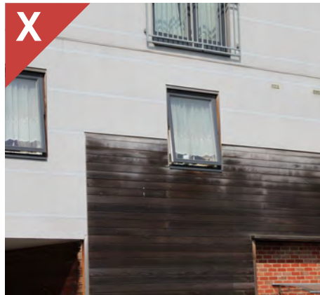
Figure 2.23i: Use of wood that weathers unevenly near material joins and has not been properly maintained.
