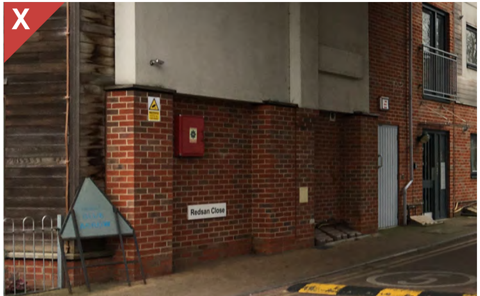
Figure 2.27a: Poorly coordinated placement of visible ancillary items on elevation visible from the street has a negative impact on the building's appearance.
